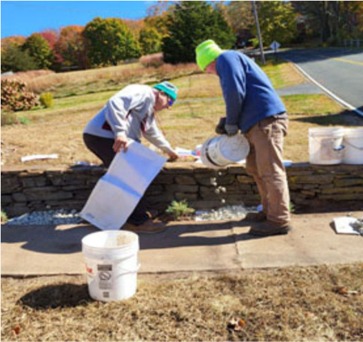
Bruce Dinnie & son Brian work on the walkway in front of the farmhouse.
